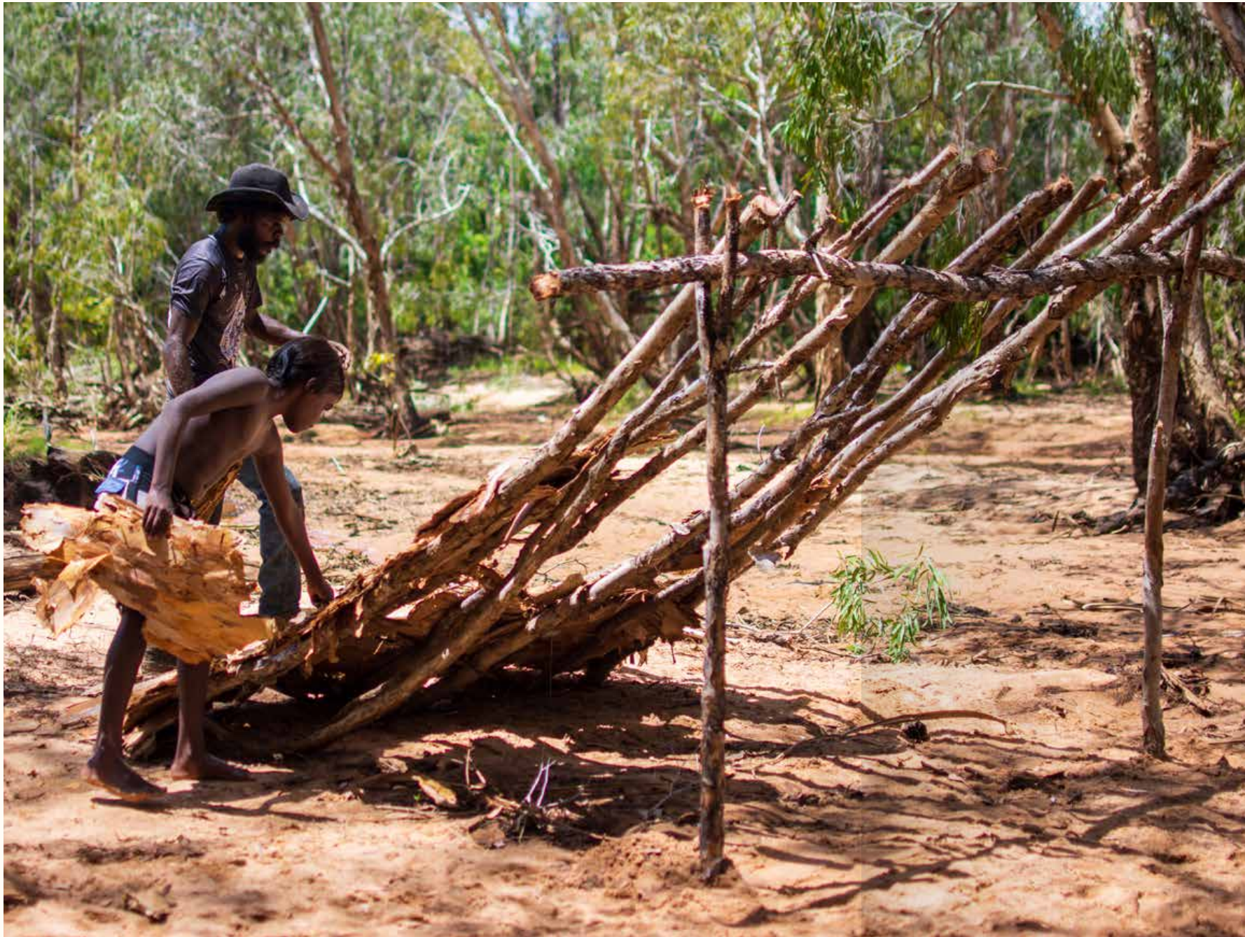
Left: A kodbarre bush shelter under construction. Some students' grandparents and great grandparents would have camped in such shelters as young people.
